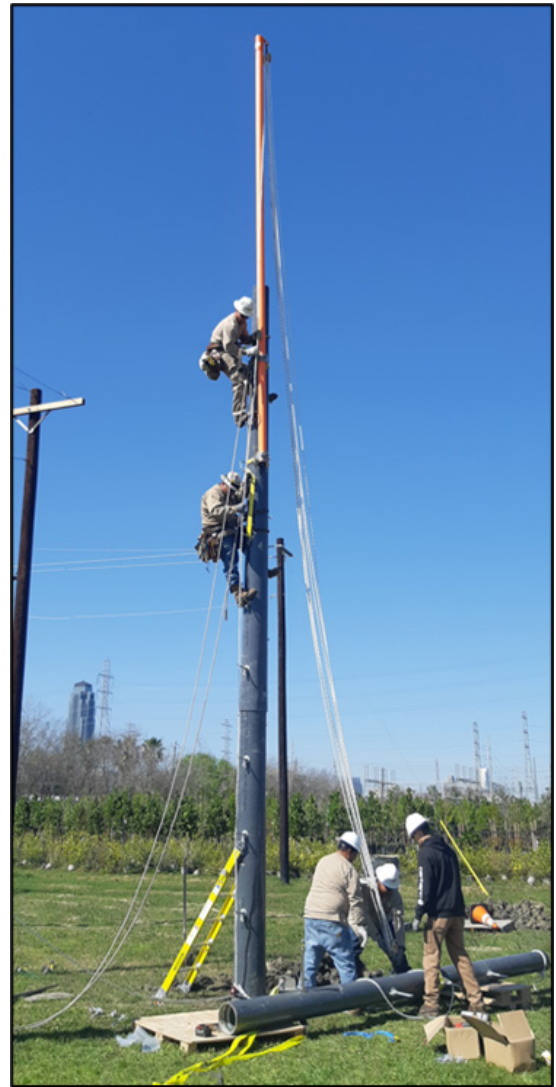
Figure 1: Line crew preparing to lift third section (RSM-02) of a 50 ft. [15.2 m] pole at a training center in Texas, USA.
