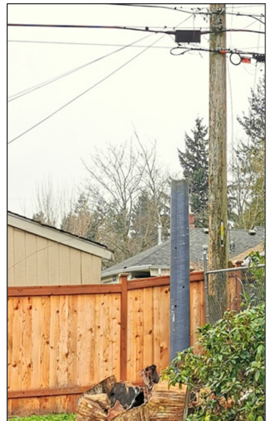
Figure 7: The base module installed in a backyard, one day prior to the planned outage.
