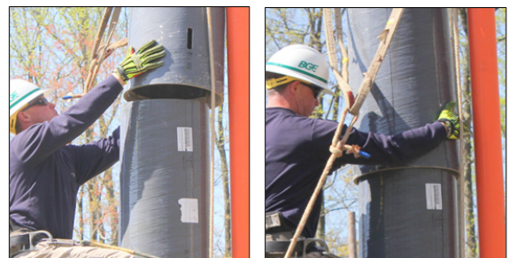
Figure 23: Keeping fingers away from pinch points, the climber gives direction to the crew while guiding the upper module onto the lower module.
