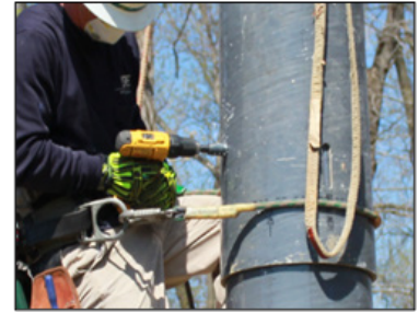
Figure 26: Chase drilling the hole for a climbing step after the joint is compressed.
