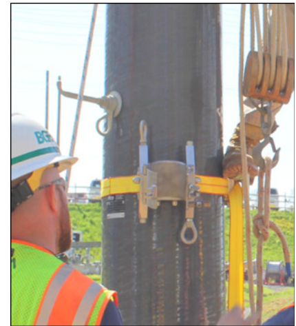
Figure 3: Climbing steps on the B and D axis; clamp assembly on the E axis, which becomes the gin axis for this installation.
