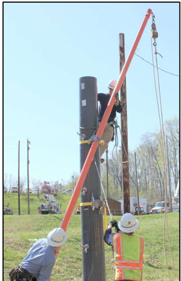
Figure 15: Sliding the gin pole through the upper clamp assembly to raise into vertical position.
