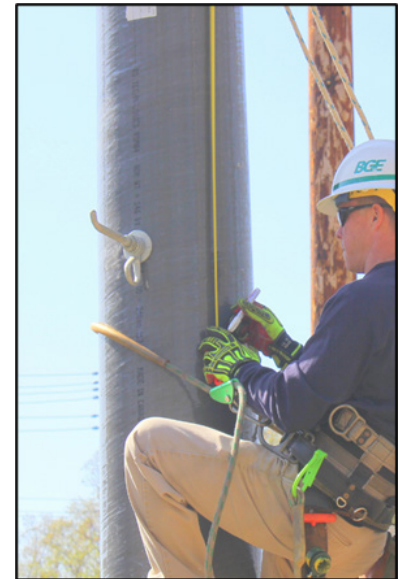
Figure 11: Measuring and marking the clamp assembly locations along the gin pole axis.
