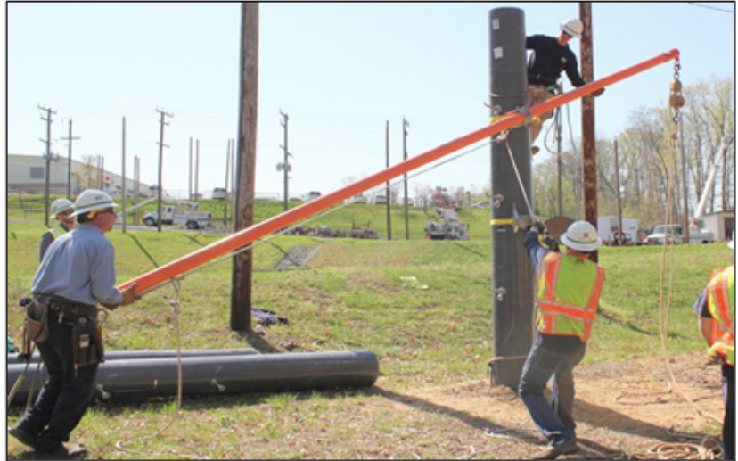
Figure 14: 3-sheave blocks and a tag line are attached to the gin head before raising the gin into the vertical position.
