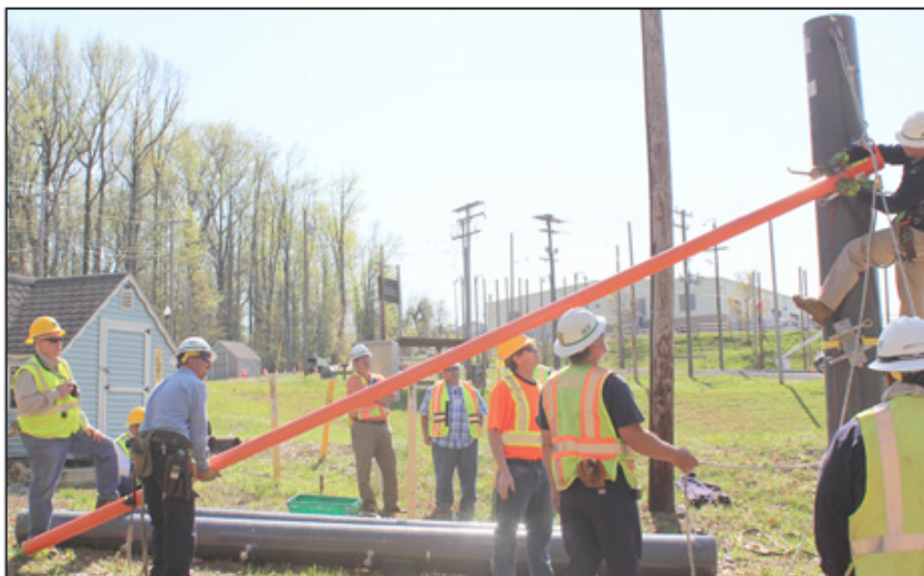
Figure 13: Climber attaches top of gin pole into the friction clamp, leaving the wing nut loose to allow the gin pole to slide into the vertical position.
