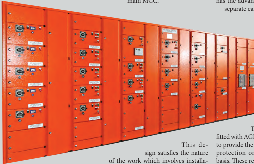
The motor control centres are manufactured to operate in harsh environments.
