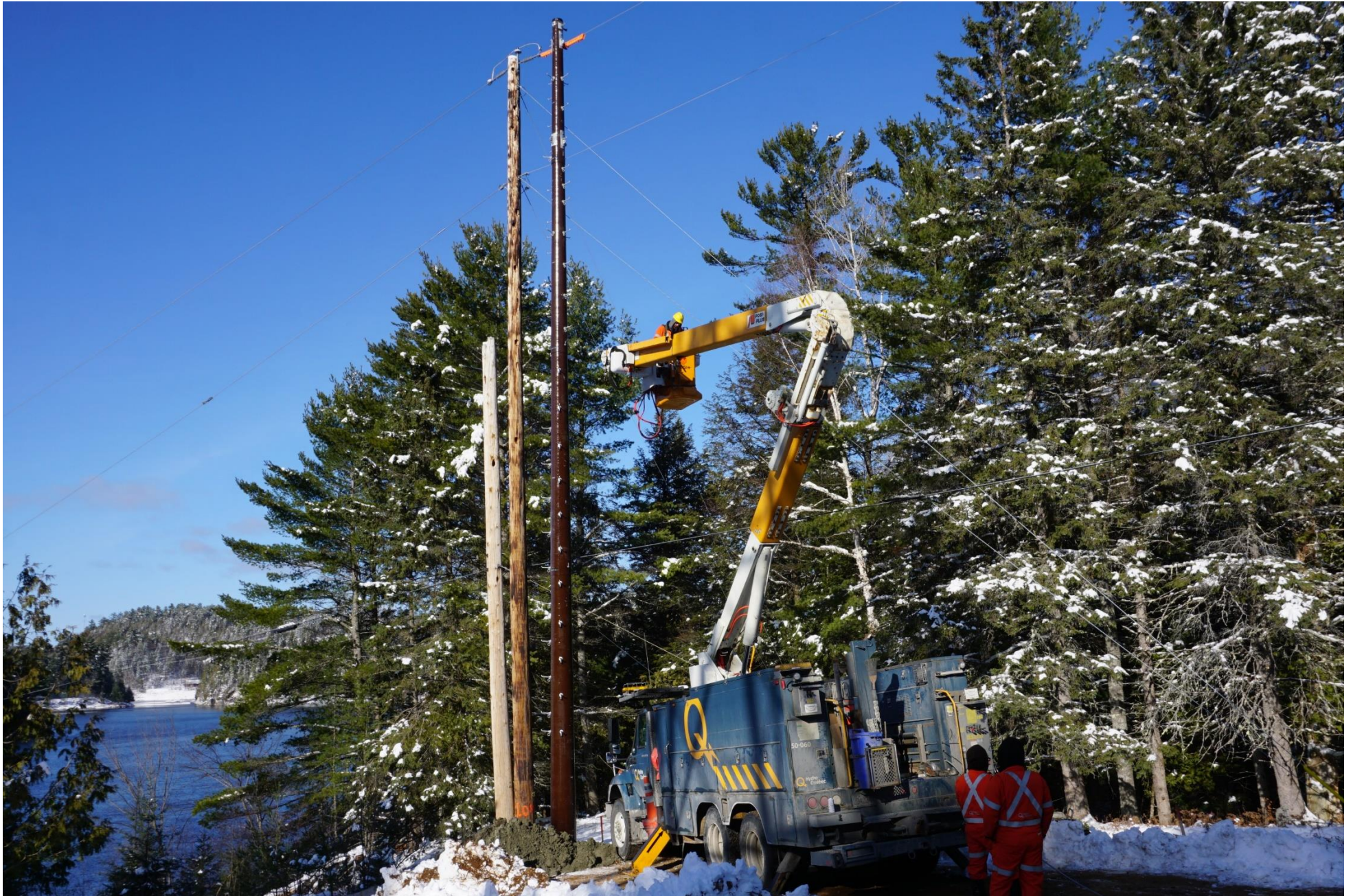
A November 2020 RS PowerON™ pole installation for a 24.9kV river crossing application by Hydro Québec north of Gatineau. Due to woodpeckers, wood pole life in this region is typically 10 years. The topped wood pole on the left is approximately 20 years old and its "like for like" replacement in the middle is about 10 years old. With the installation of the RS composite pole guarding against future woodpecker damage, utilities like Hydro Québec are proceeding confidently based on the pole's expected 80-year service life.
