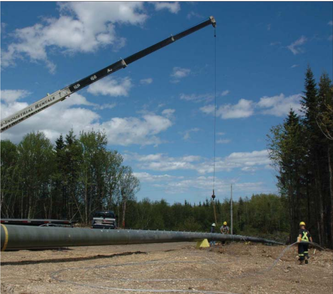
A medium-size crane is positioned to hoist a 93-foot RS Standard monopole. The installation did not require a concrete foundation. From the time the crane arrived to the time the pole was guyed into place, about one hour elapsed.
