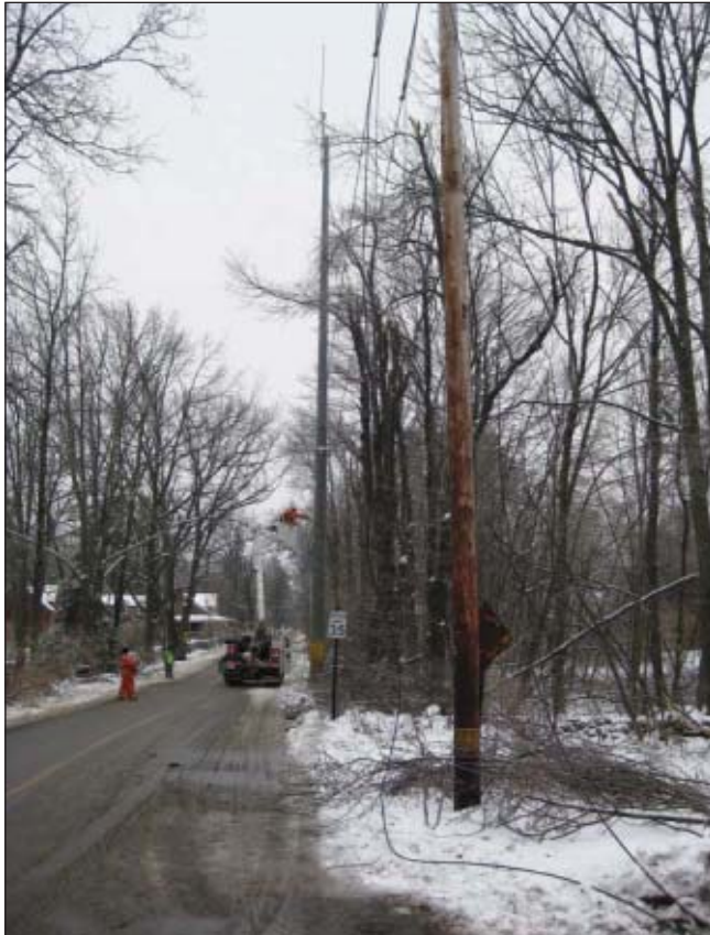
A December 2008 ice storm snapped wooden poles owned by the Princeton, Mass., Municipal Light Department, but not their dual-use composite poles. The 75- to 80-foot composite poles were used for both electric power delivery and top-mounted broadband antennas.
