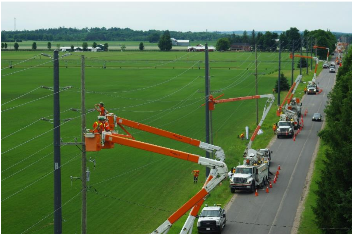
RS Composite Utility Poles Installation for a Hydro One 44kV Grid Hardening Project
