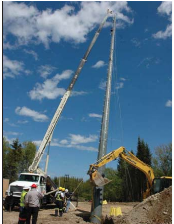
This May 2009 composite RS monopole installation in Nova Scotia provides an example of fast, direct-bury installations. These poles saved thousands of dollars by not requiring foundation materials and by speeding installation — only a crane and a backhoe were used.
