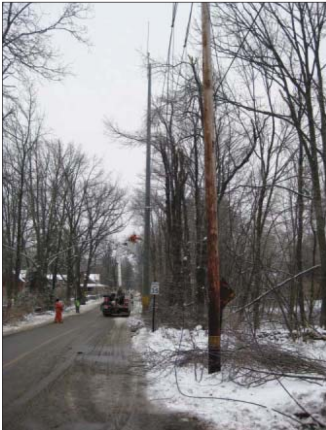
A December 2008 ice storm snapped wooden poles owned by the Princeton, Mass., Municipal Light Department, but not their dual-use composite poles. The 75- to 80-foot composite poles were used for both electric power delivery and top-mounted broadband antennas.
