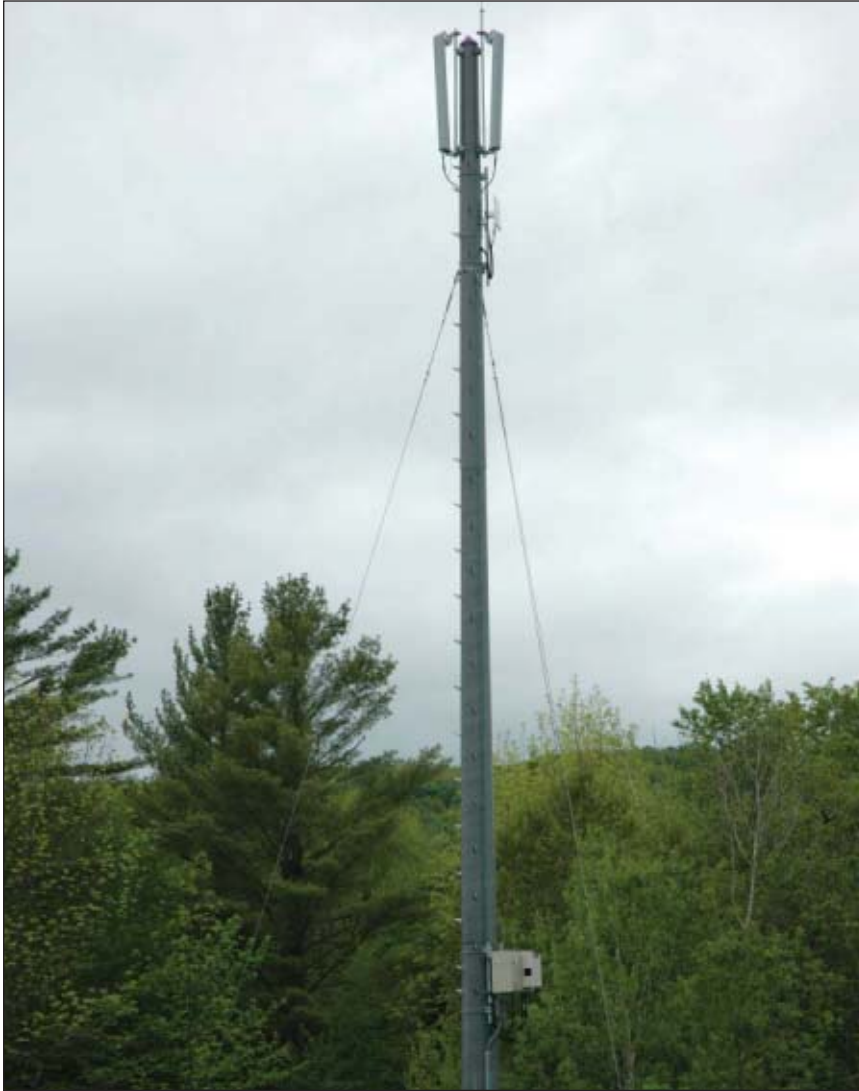
In Dalton, N.H., NCIC installed an RStandard monopole on land donated by the owner of the site so her neighbors could have broadband access.
