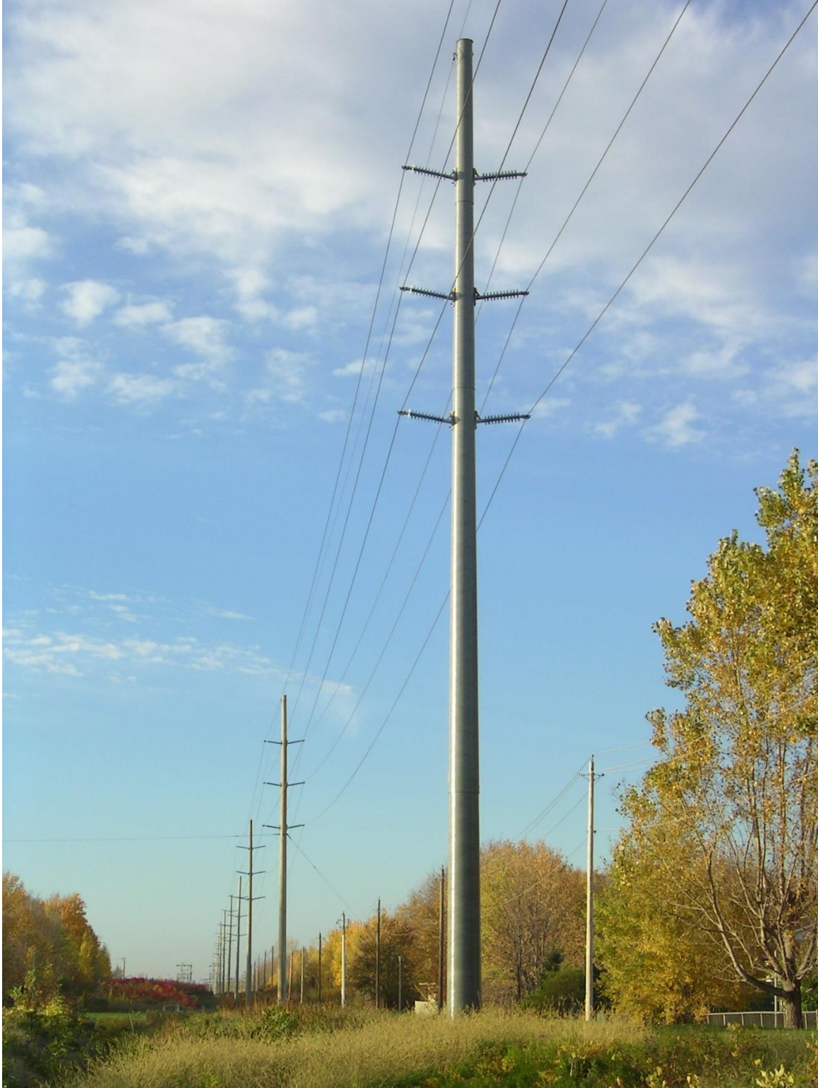
Double circuit 115kV RS pole installed with Cornwall Electric (A FortisOntario Company) in Cornwall, Ontario, Canada
