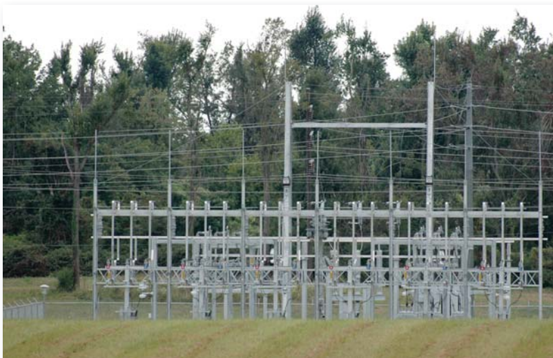
A composite pole was used for a 69-kV transmission switch pole connection into a new distribution substation.
