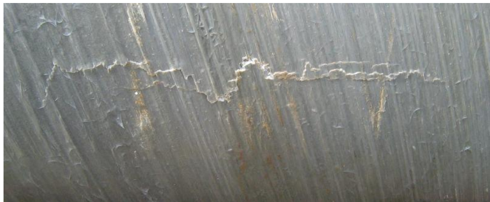
Figure 6 - Structural Damage, Mishandling
