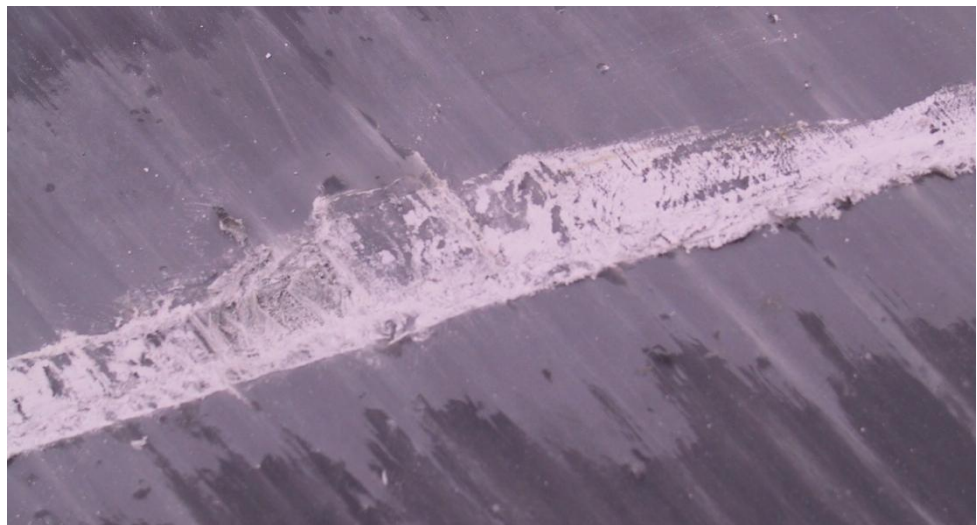
Figure 4 - Surface Damage Gouge (intervention required)
