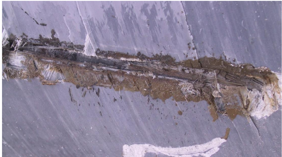
Figure 5 - Structural Damage, forklift penetration
